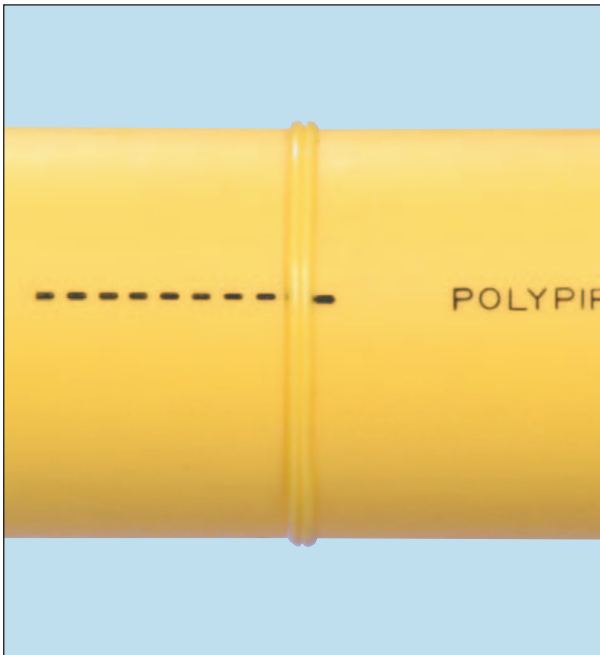
Melt bead too small due to insufficient heat time.
